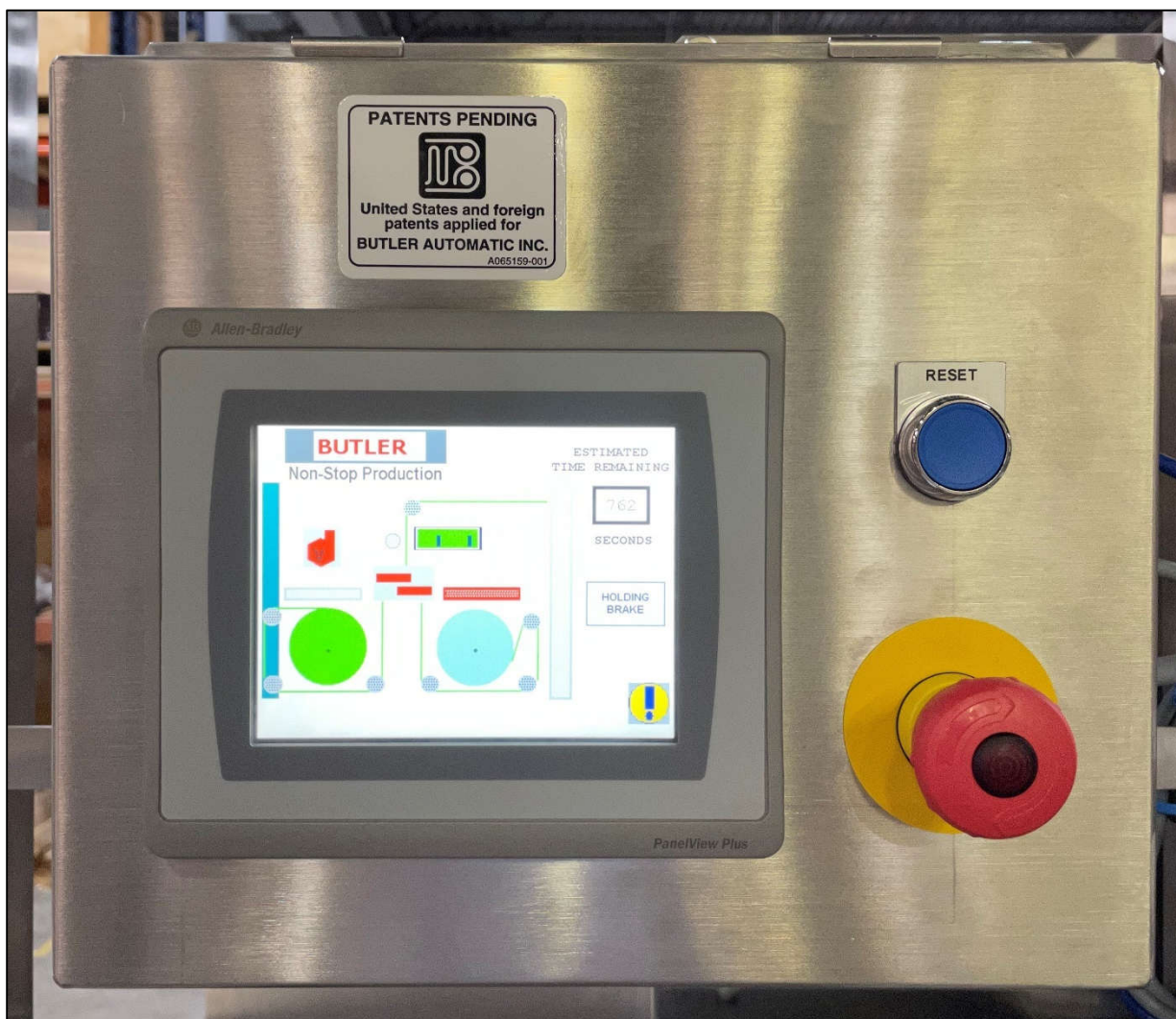
OPERATOR INTERFACE PANEL
