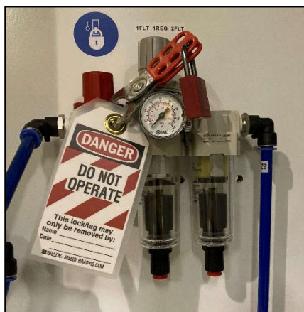
Pneumatic System Locked Out
