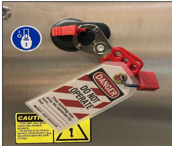
MAIN POWER SWITCH LOCK-OUT
